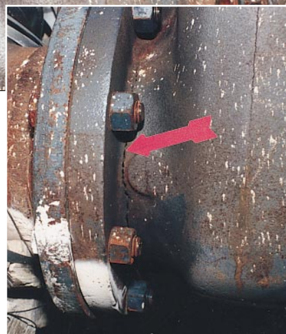
5 Pit 3a 8-in. cast-iron gate valve. Note the crack extending around circumference of flange neck.
