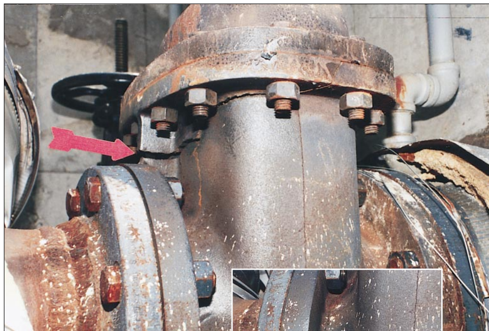
4 Pit 3a 8-in. cast-iron gate valve. Note the broken gusset.
