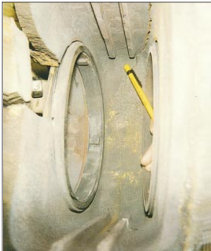
8 Inside of Pit 3a valve. Pencil points to valve disk guides.
