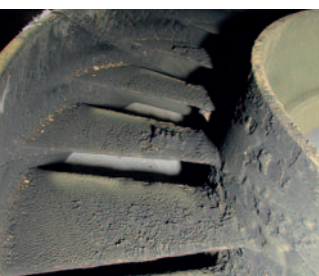
Components are sufficiently clean: no changes needed.
