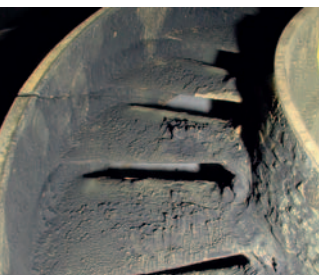
Components too dirty: shorten cleaning intervals.
