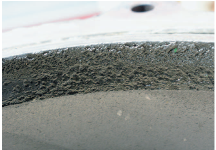
Layer of scale deposited on a turbine diffuser
