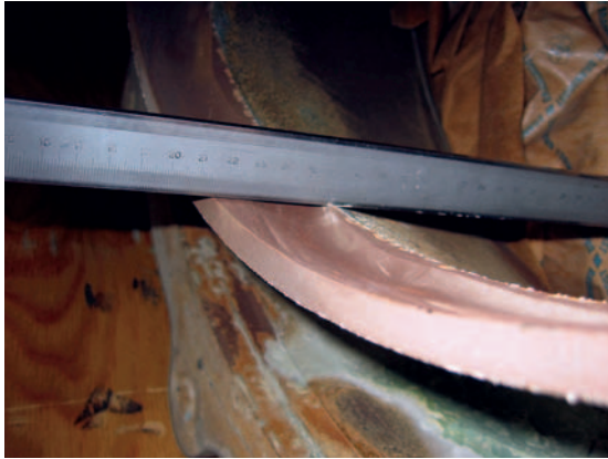
Worn turbine diffuser.
