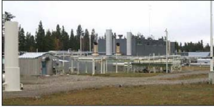
A Compressor Station
