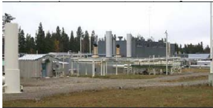
A Compressor Station
