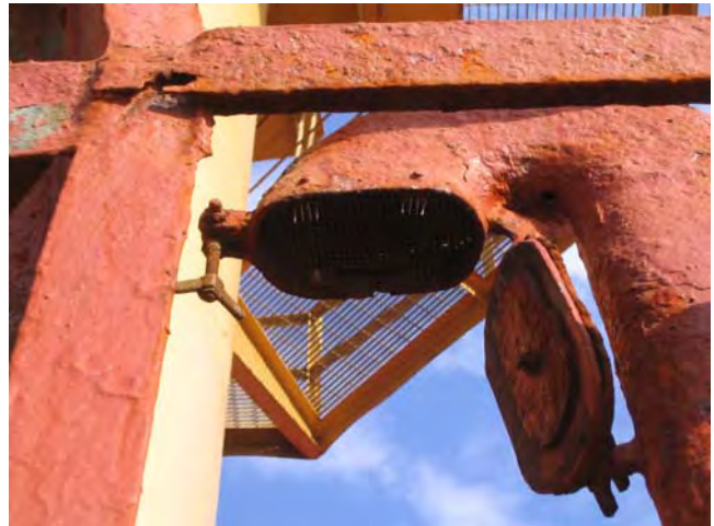
Wasted gooseneck ventilator
