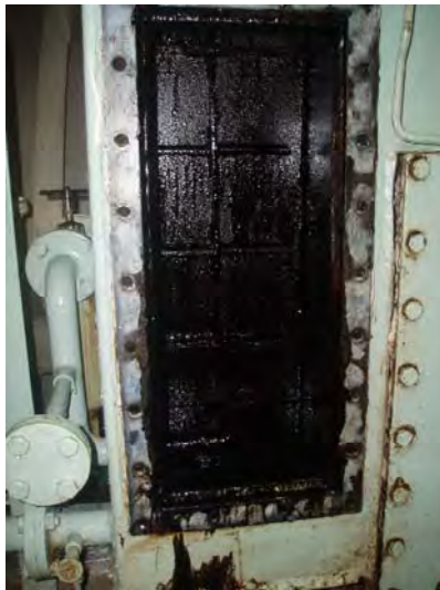
Oily inside of oil water separator
