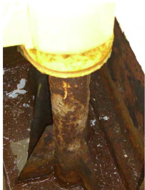
Corrosion of air pipe
