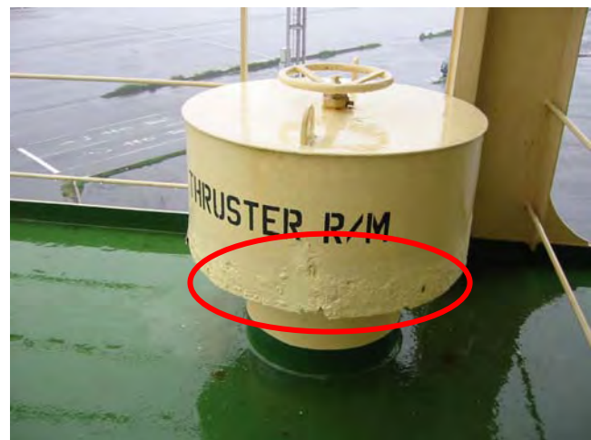
Wastage of the casing of ventilator
