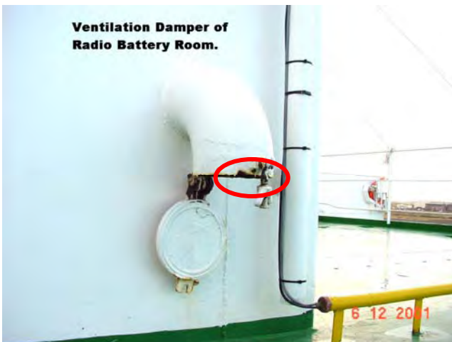
Wasted wall ventilator
