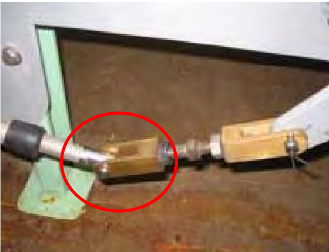
Incorrect condition of turn buckle
