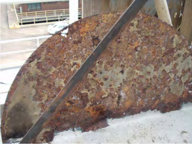
Wastage/holes of fire damper
