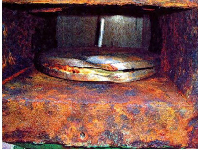
Damage of disk float
