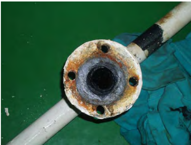
Oily inside of discharge pipe
