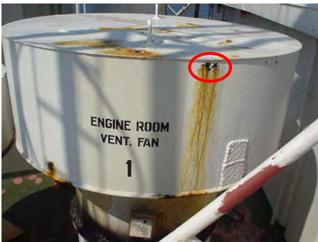
Holes of the casing of ventilator
