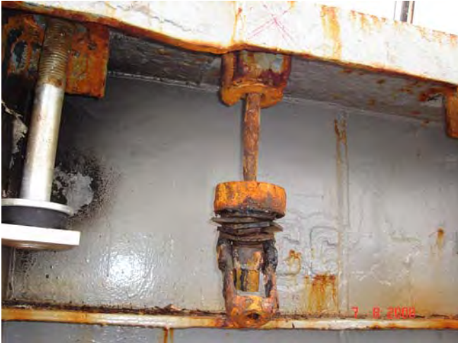
Wasted securing device
