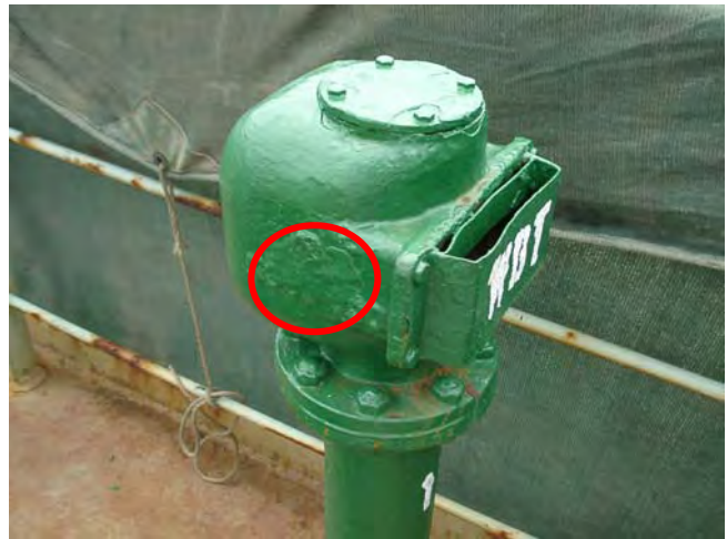
Temporary repaired by patty → Not acceptable!
