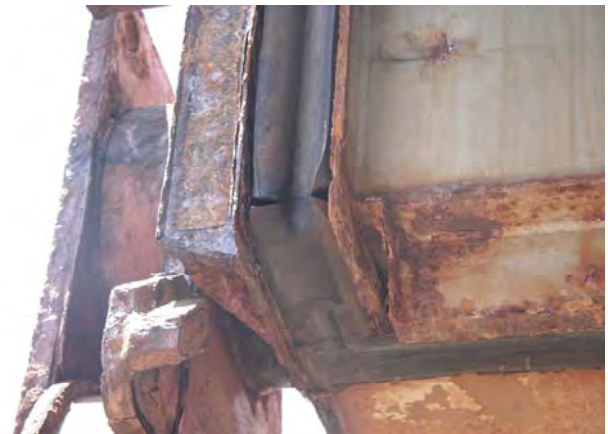
Deteriorated and cracked rubber packing
