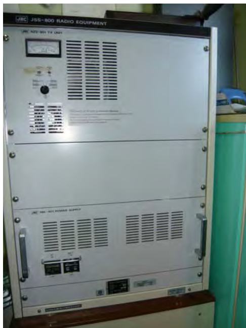
Switch Panel for MF/HF radio
