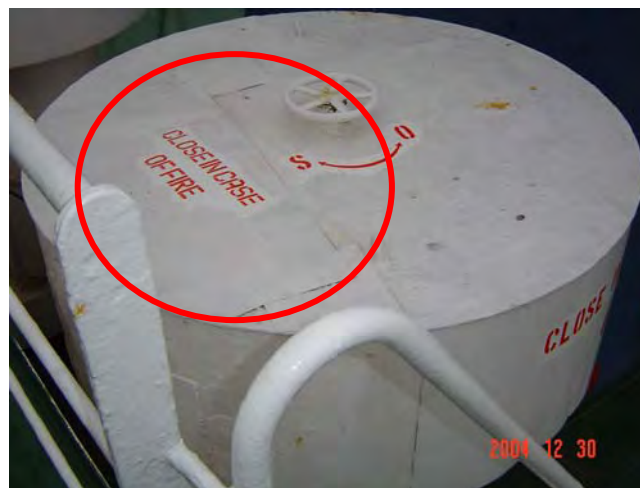
Temporary repair by tape → Not acceptable!
