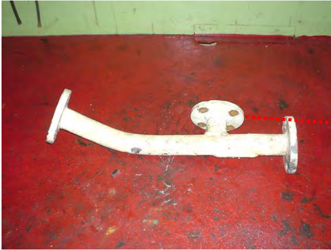
Flange connection to by-pass line
