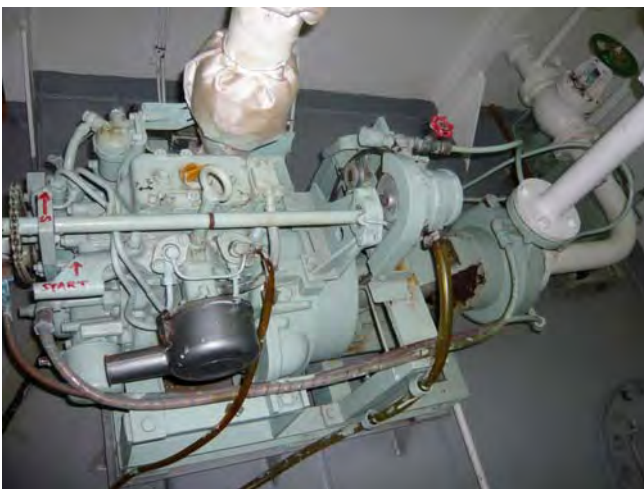
Emergency fire pump
