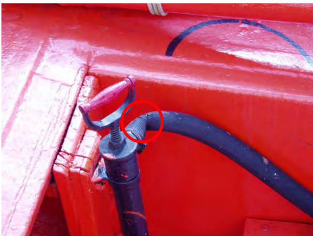
Cracked hose of bilge pump
