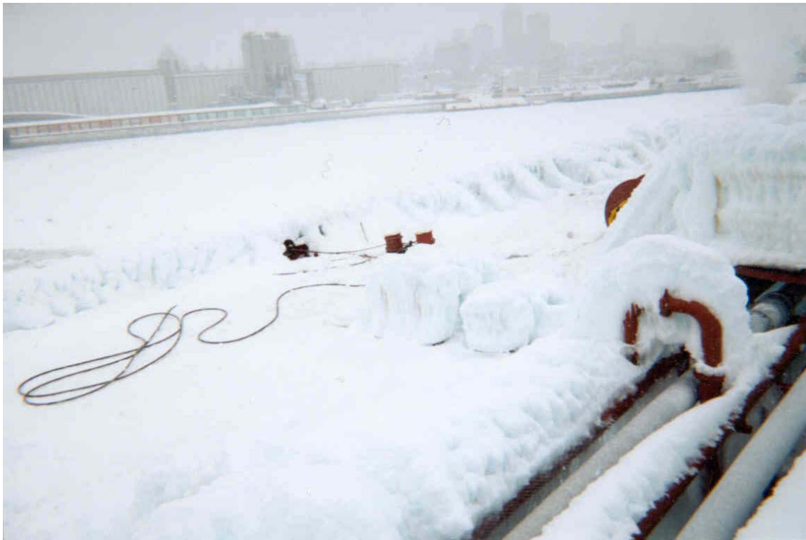
Figures 5.3F– Deck, piping and valves inaccessible
