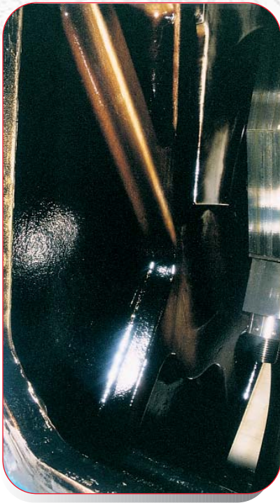
Figure 9: Conventional type lubricant; typical crankcase blackening as a result of heavy fuel contamination of lubricant
